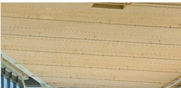
Figure 54: Sprinkler pipes and nozzles suspended from a Kerto-Q panel.
