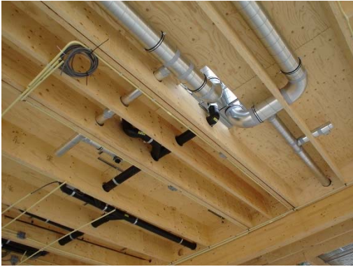
Figure 27: Ventilation channels and water pipes in an intermediate floor made of Kerto.
