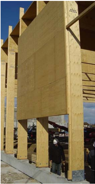
Figure 22: A hall braced with Kerto-Q panels.
