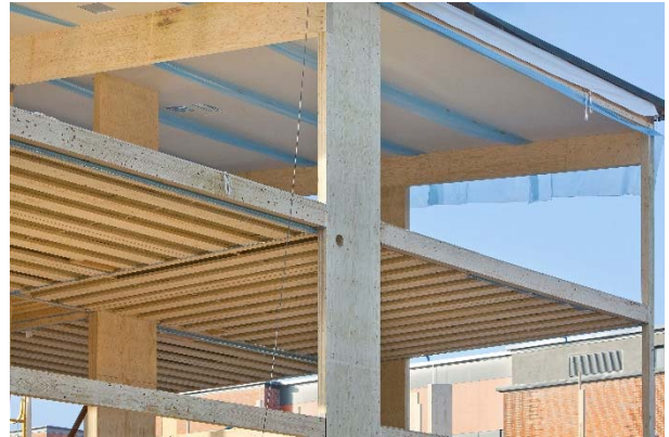
Figure 39: Kerto-Ripa elements in the floor structure of an apartment building and massive glued Kerto-Q columns.
