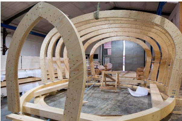
Figure 36: Kerto-Q arches for the roof structure of a windmill. The structure consists of several curved members.
